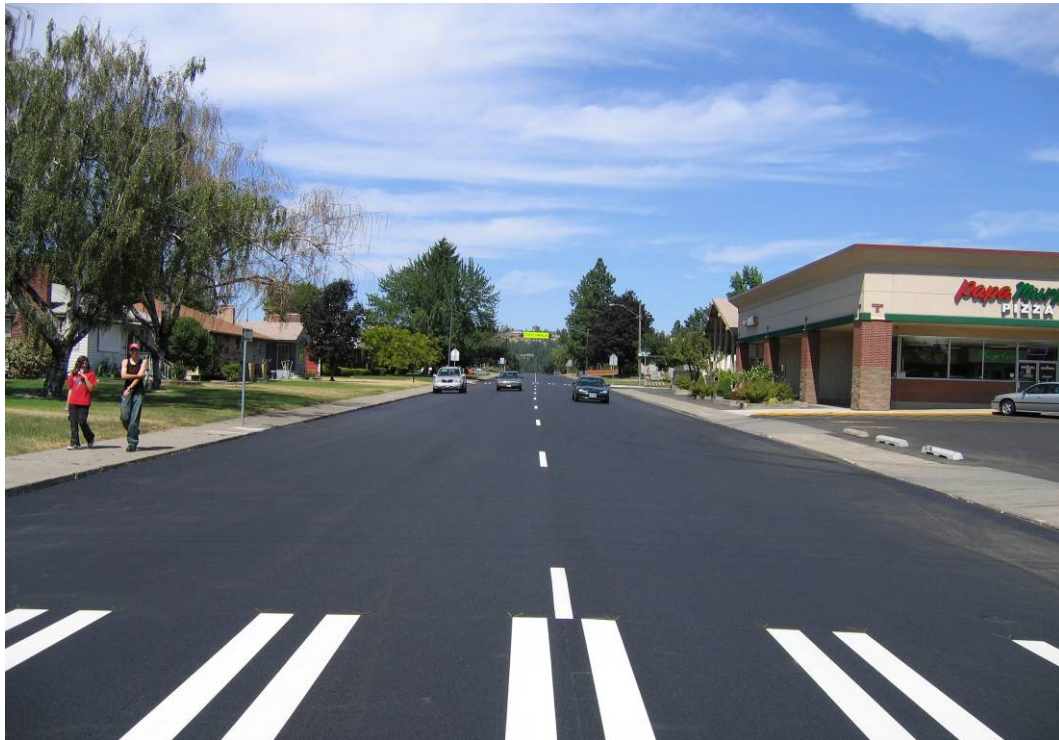
Southbound Ash Street just north of Rowan Avenue after completion of construction.
